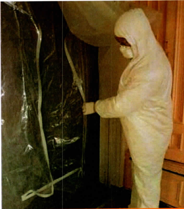
Plastic sheeting helps prevent tracking dust and debris out of the work area.
