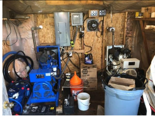
Generator Building (1) 10KW & (1) 20KW
