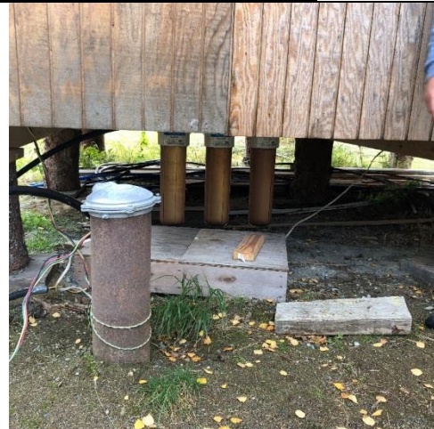
Well / Filter system
