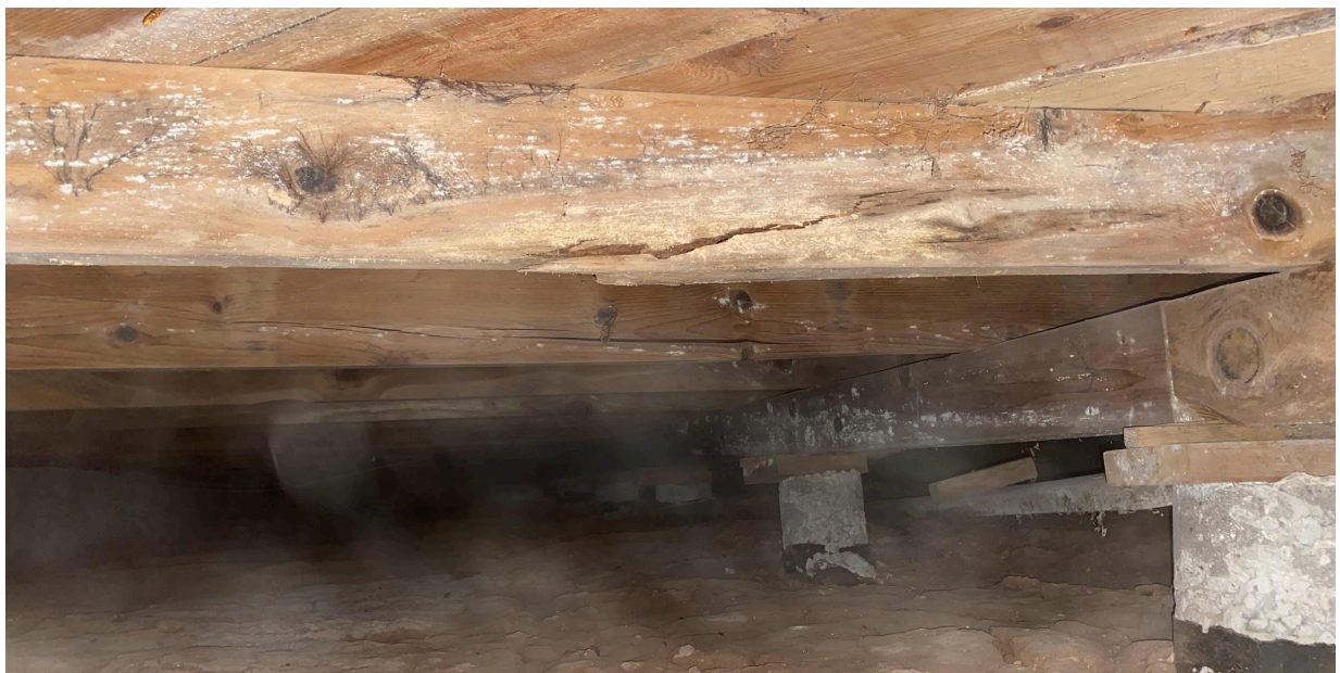
Damaged floor joist in need of repair.
