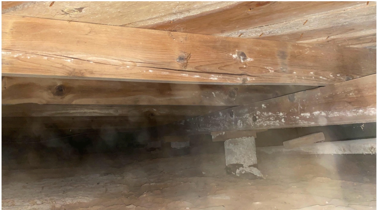
Damaged floor joist in need of repair.
