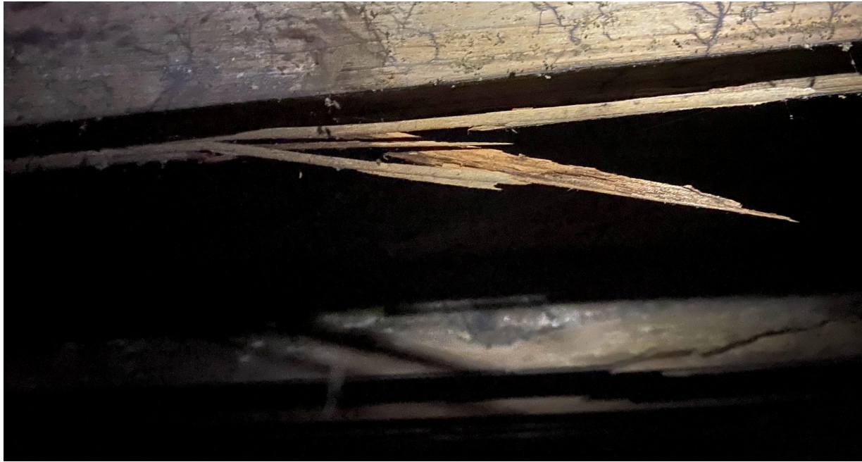
Dry rotted floor joist in need of repair.
