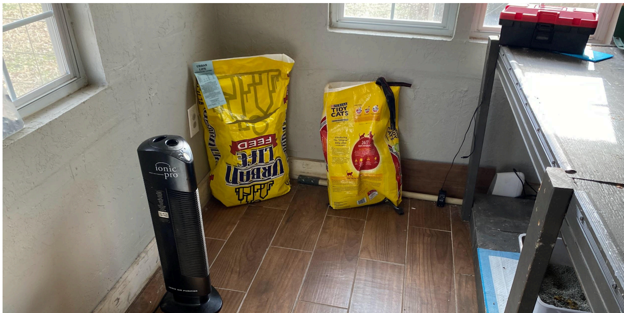
Backroom add-on's concrete floor slopes but did not see cracking or separation in the add-on's structure.
