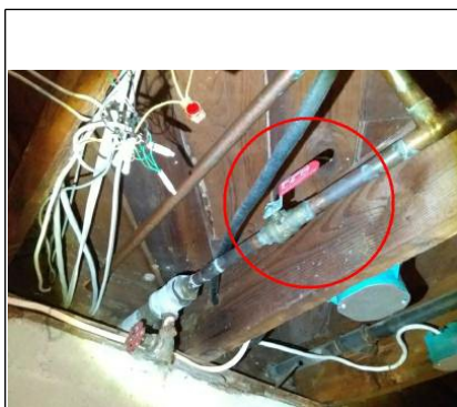
Water main shut off valve
