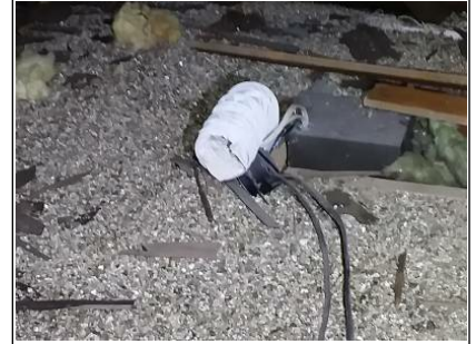
East hallway Bathroom exhaust vent
